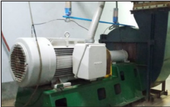
Ventilation fan motors operating at 3600 RPM.
